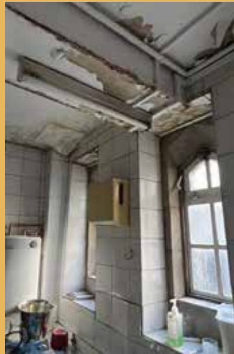
CONDEMNED KITCHEN WITH WATER INGRESS
