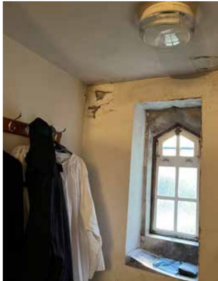
WATER INGRESS IN THE SACRISTY
